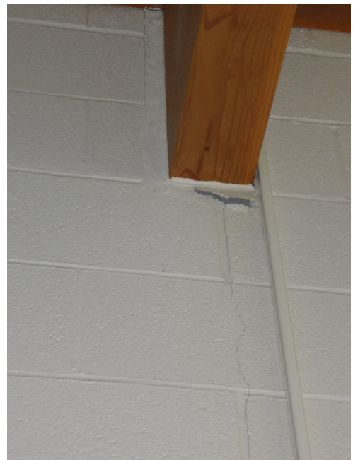
36. ENLARGED IMAGE OF MASONRY CRACK OBSERVED ON WEST WALL OF ROOM 19 – ART. - CONSULT STRUCTURAL ENGINEER TO MONITOR AND DETERMINE REPAIR SOLUTION
