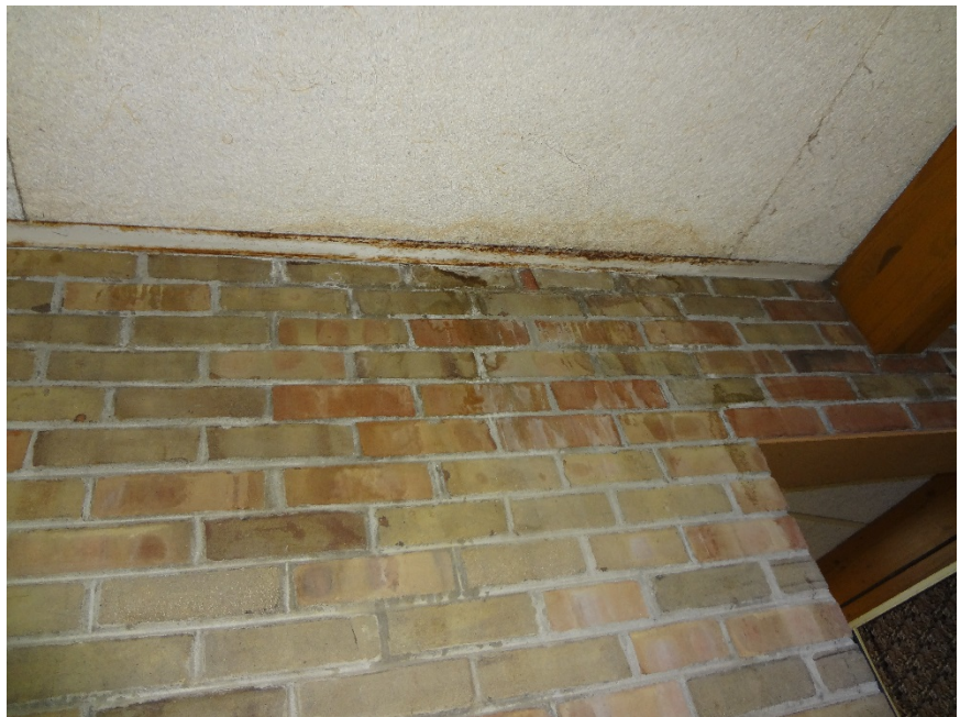
38. CORROSION OF METAL FRAMING, STAINING FROM MOISTURE INFILTRATION - INVESTIGATE SOURCE OF MOISTURE AND REPAIR. CLEAN BRICK AND CEILING ASSEMBLY
