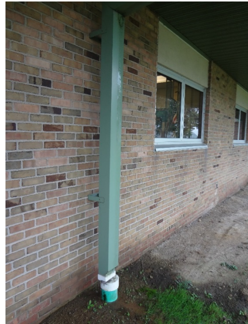
16. ANOTHER DOWNSPOUT LEAKING FROM SEAM AT TOP OF DOWNSPOUT - CLEAN, INSPECT AND REPAIR DOWNSPOUT CONNECTION AS REQUIRED
