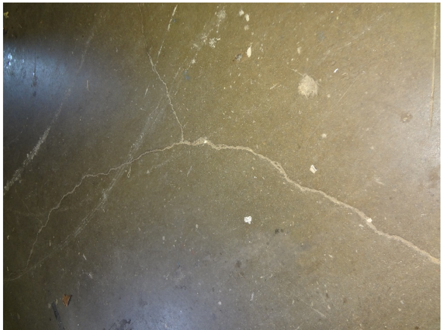
27. CRACKING IN CONCRETE FLOOR THROUGHOUT STORAGE AREA - CRACKING IS INHERENT IN CONCRETE. MONITOR FOR MOVEMENT, FINISH IF DESIRED
