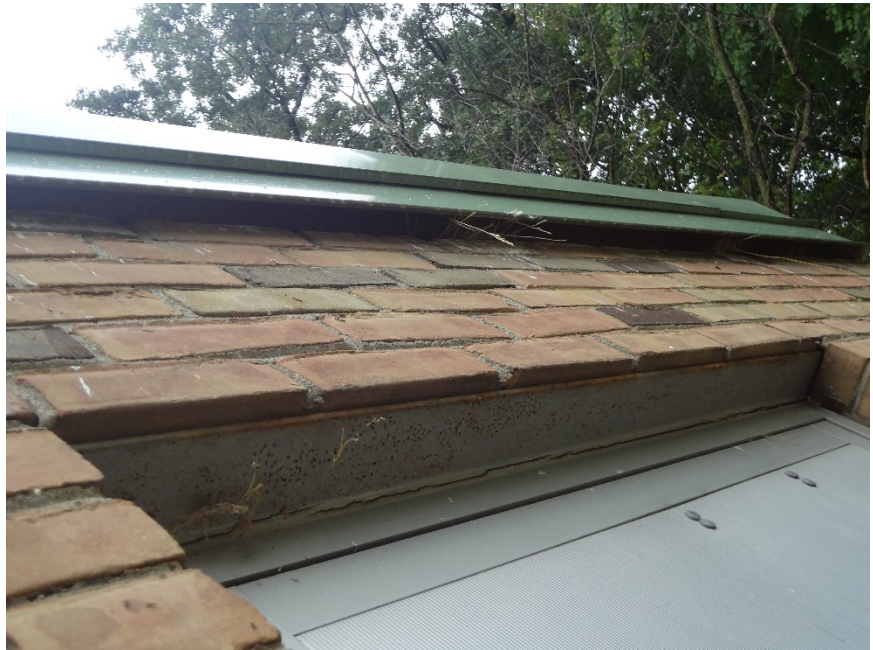
31. WIDE OPENING AT METAL ROOF FLASHING ALLOWING WEATHER INFILTRATION + NESTING - CLEAN DEBRIS FROM OPENING AND INFILL FLASHING TO CLOSE AREA OF INFILTRATION
