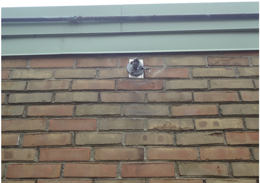
34. BROKEN EXTERIOR LIGHT FIXTURE ARM + MISSING EXTERIOR LIGHT FIXTURE - REPLACE EXTERIOR LIGHT FIXTURE
