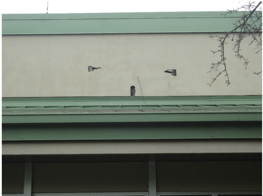
10. PUNCTURES IN EIFS, ALLOWING AIR + WATER INFILTRATION INTO ROOF CAVITY - PATCH AND REPAIR EIFS, FINISH TO MATCH EXISTING
