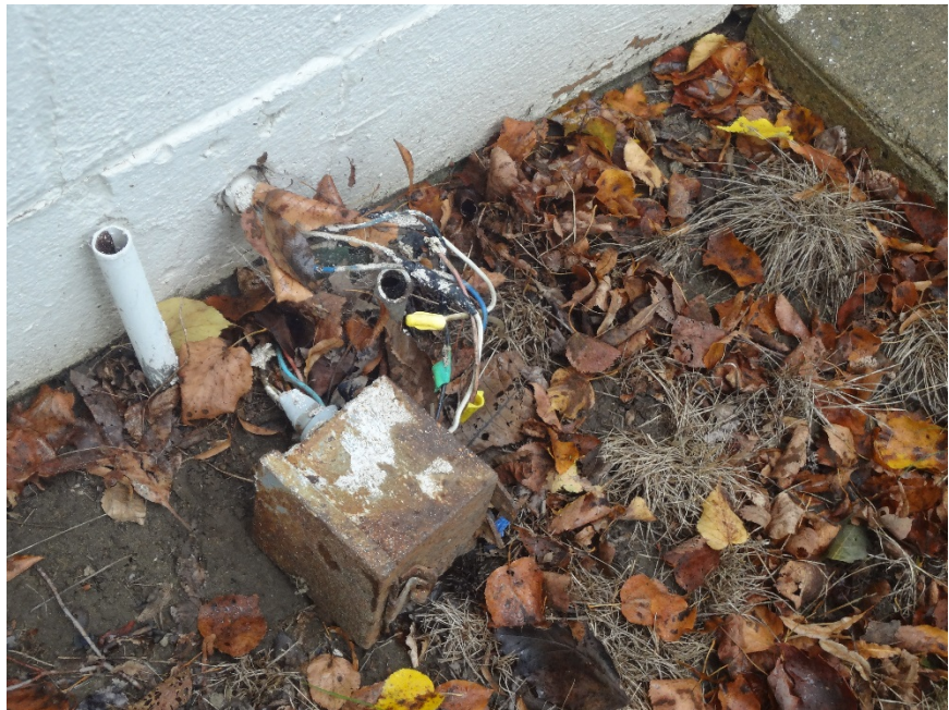
11. BROKEN CONDUIT + EXPOSED WIRING OF ABANDONED JUNCTION BOX - DISCONNECT JUNCTION BOX AND CAP ELECTRICAL AS REQUIRED
