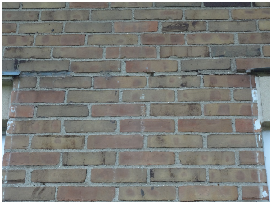
4. ERODED + LOOSE GROUT, TYPICAL AT DOOR + WINDOW FLASHING - CLEAN & REPOINT MASONRY AS NEEDED FOR DAMAGED JOINTS. INSPECT ANNUALLY.
