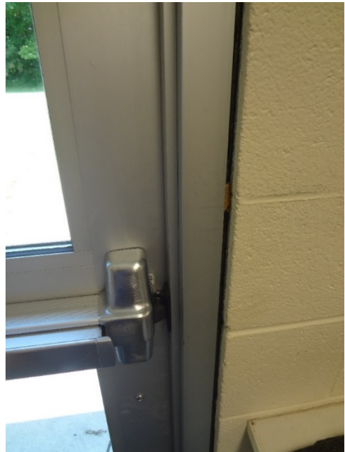
40. ENLARGED IMAGE OF MISSING BACKER ROD + SEALANT AROUND DOOR FRAME - INSTALL BACKER ROD AND CAULK AROUND FRAME, INSPECT WEATHERSTRIPPING
