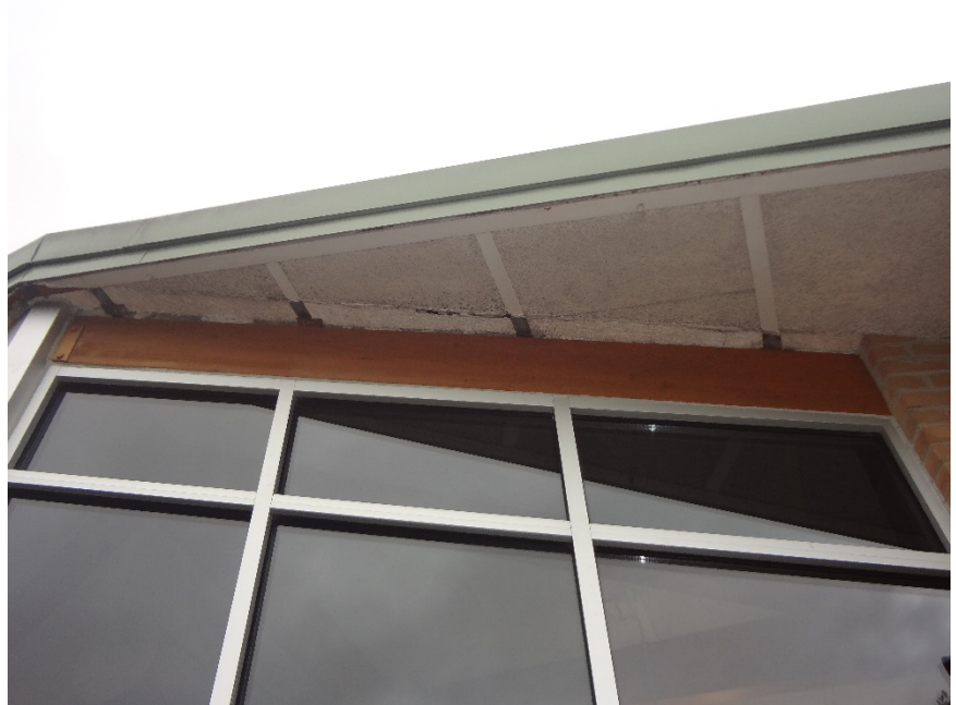
32. MISSING TRIM AT TECTUM SOFFIT EXPOSING STRUCTURE TO CORROSION + INFILTRATION - REPLACE METAL SOFFIT TRIM AND ENSURE OPENING IS WEATHER TIGHT
