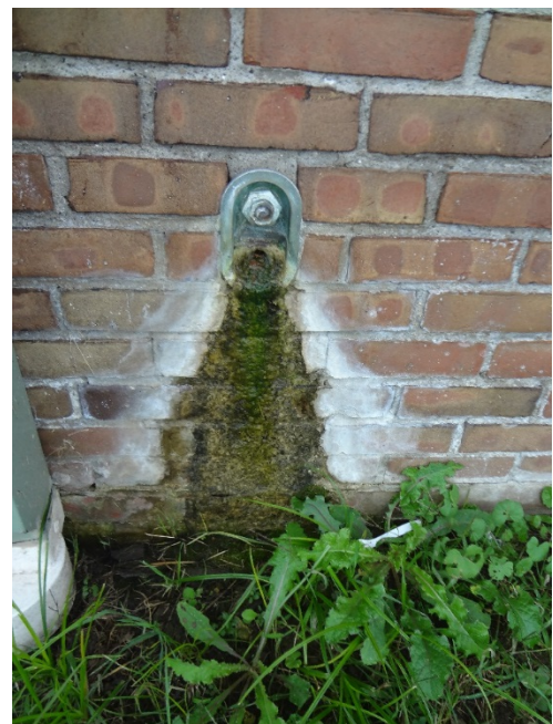
12. ORGANIC GROWTH + STAINING BELOW BROKEN WATER BIB - CLEAN ORGANIC MATTER FROM BRICK, INSPECT WATER BIB AND REPAIR AS REQUIRED
