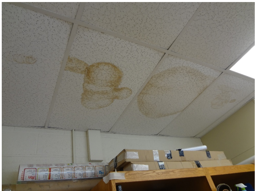
25. WATER STAINED CEILING TILES INDICATE A POTENTIAL OF WATER INFILTRATION AT ROOF - INVESTIGATE SOURCE OF MOISTURE AND REPAIR. REPLACE CEILING TILES
