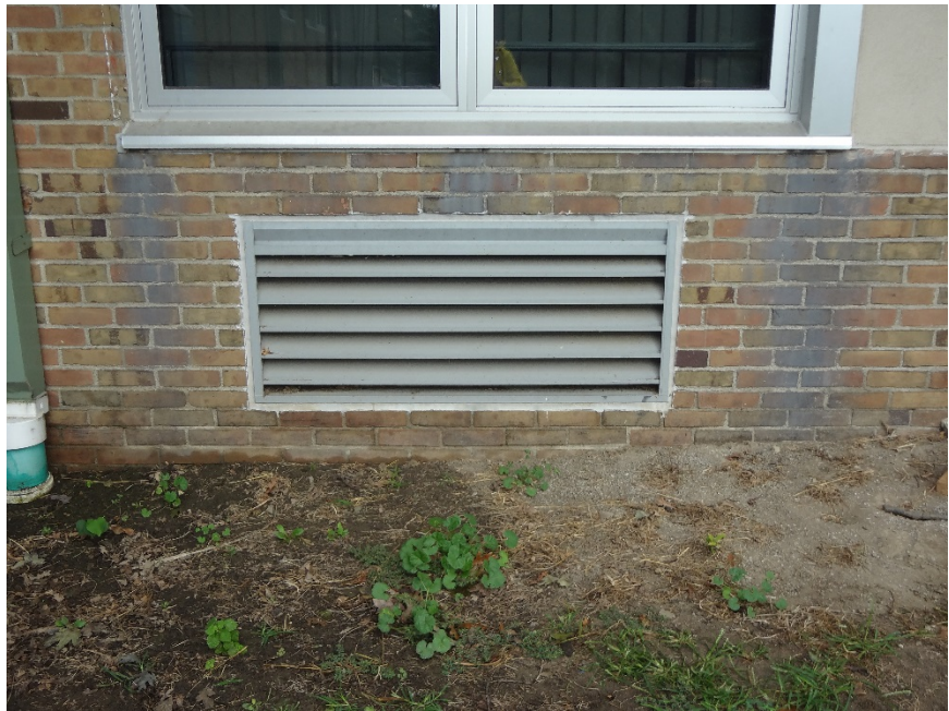
7. ALUMINUM STAINS ON BRICK, TYPICAL AT ALL WINDOWS THROUGHOUT FACILITY - CLEAN AND SEAL MASONRY AS NEEDED IN ALL SIMILAR LOCATIONS.
