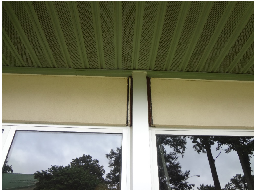
9. PLYWOOD + GYPSUM BOARD EXPOSED TO EXTERIOR ELEMENTS - CUT-BACK PLYWOOD AND GYPSUM, INFILL OPENING FOR WEATHER TIGHTNESS
