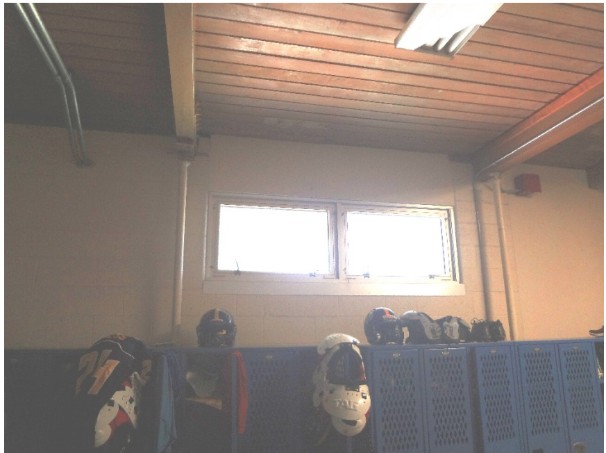
22. TWO RETROFIT STEEL JACKPOSTS AT LAMINATED WOOD BEAMS - CONSULT STRUCTURAL ENGINEER. TO BE REPAIRED/REPLACED DURING 2019 REMODEL
