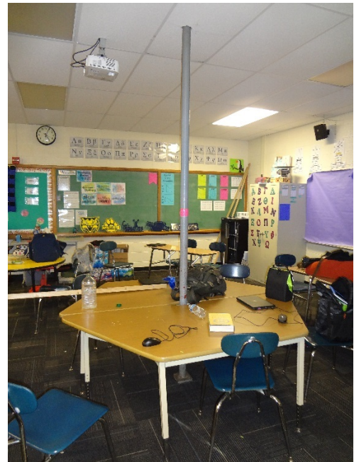
28. RETROFIT STEEL JACKPOST AT CENTER OF CLASSROOM - CONSULT STRUCTURAL ENGINEER TO MONITOR AND DETERMINE REPAIR SOLUTION
