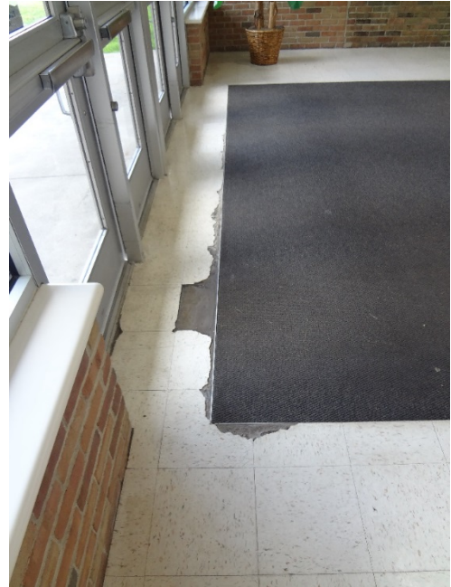
18. BROKEN VCT AT VESTIBULE ENTRY FROM WATER INFILTRATING UNDER DOORS, TYPICAL - STOP WATER INFILTRATION. FLOOR REPLACEMENT IN 2019, PART OF SINKNG FUND PROJECT
