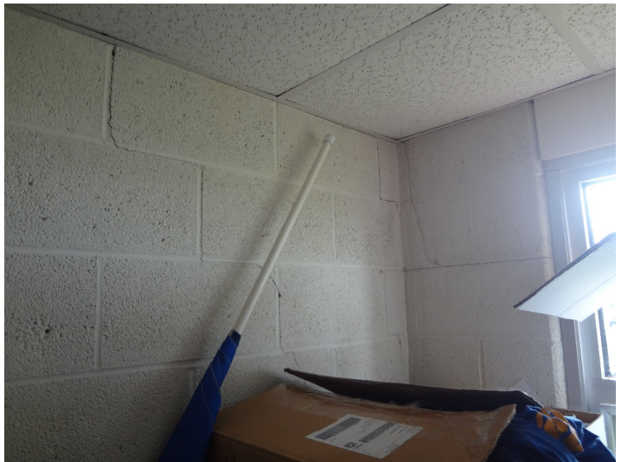
21. MASONRY CRACKS THROUGHOUT SOUTHEAST CORNER OF STORAGE ROOM - CONSULT STRUCTURAL ENGINEER TO MONITOR AND DETERMINE REPAIR SOLUTION
