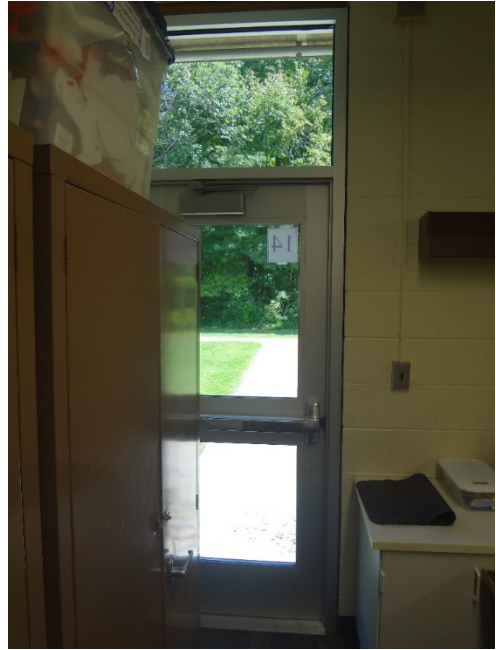
39. MISSING BACKER ROD + SEALANT AROUND ENTIRE DOOR FRAME - INSTALL BACKER ROD AND CAULK AROUND FRAME, INSPECT WEATHERSTRIPPING
