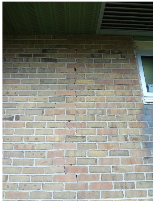
6. BROKEN + MISSING BRICK + ERODED GROUT THROUGHOUT AREA OF FAÇADE - CLEAN & REPOINT MASONRY AS NEEDED FOR DAMAGED JOINTS. INSPECT ANNUALLY.
