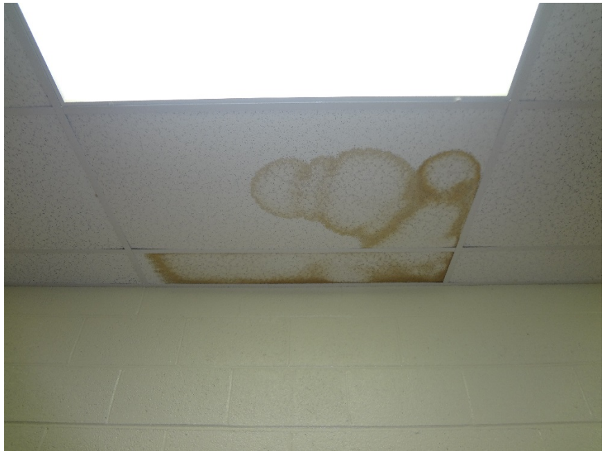
30. WATER STAINED CEILING TILES INDICATE A POTENTIAL OF WATER INFILTRATION AT ROOF - INVESTIGATE SOURCE OF MOISTURE AND REPAIR. REPLACE CEILING TILES
