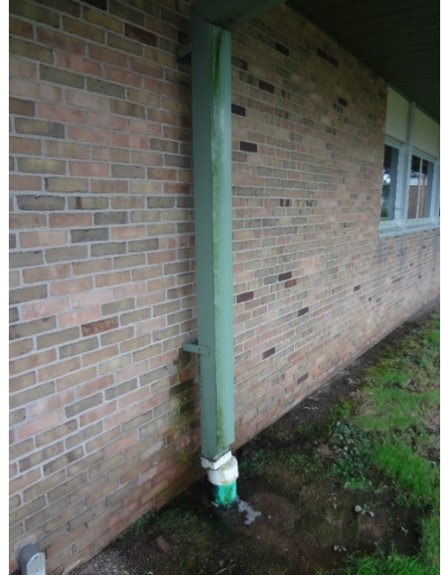
15. WATER LEAKING FROM TOP OF DOWNSPOUT, ORGANIC GROWTH ON FACE - CLEAN, INSPECT AND REPAIR DOWNSPOUT CONNECTION AS REQUIRED
