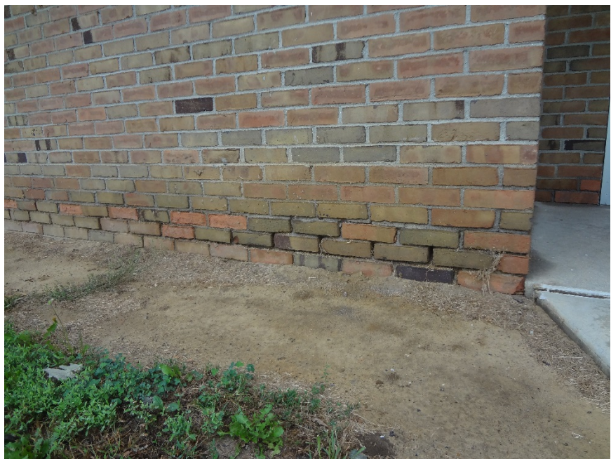
8. BROKEN + ERODED GROUT, 2'-0" ABOVE GRADE AND BELOW, TYPICAL - CLEAN & REPOINT MASONRY AS NEEDED FOR DAMAGED JOINTS. INSPECT ANNUALLY.
