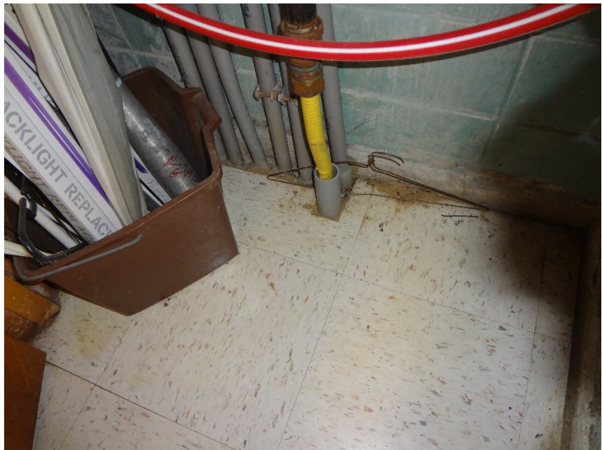
24. AREA OF WATER AND SAND INFILTRATION INTO CLASSROOM DURING HEAVY RAINS - CAMERA (INSPECT) UNDERGROUND STORM LINE TO DETERMINE CAUSE, REPAIR
