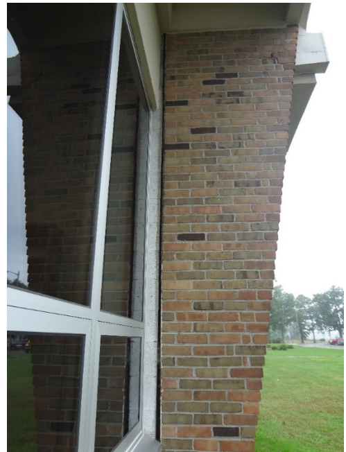
14. OPEN EXPANSION JOINT, SHOULD BE FILLED WITH BACKER ROD + SEALANT - INSTALL BACKER ROD AND CAULK AROUND FRAME, INSPECT WEATHERSTRIPPING
