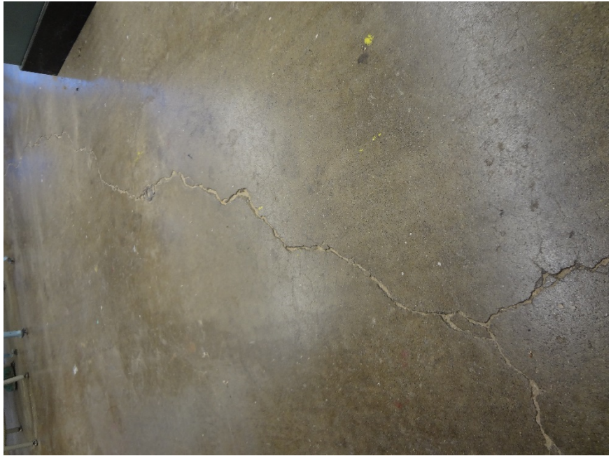
26. CRACKING IN CONCRETE FLOOR THROUGHOUT SHOP AREA - CRACKING IS INHERENT IN CONCRETE. MONITOR FOR MOVEMENT, FINISH IF DESIRED
