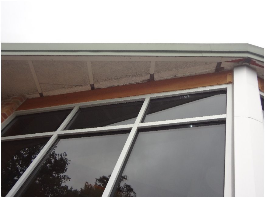
33. MISSING TRIM AT TECTUM SOFFIT EXPOSING STRUCTURE TO CORROSION + INFILTRATION - REPLACE METAL SOFFIT TRIM AND ENSURE OPENING IS WEATHER TIGHT
