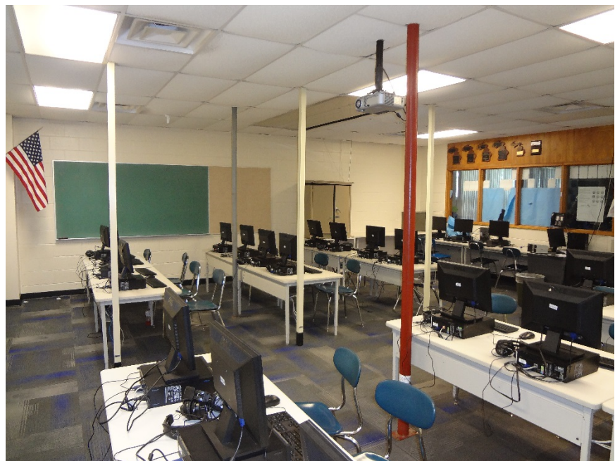
29. TWO RETROFIT STEEL JACKPOSTS AT CENTER OF COMPUTER LAB - CONSULT STRUCTURAL ENGINEER TO MONITOR AND DETERMINE REPAIR SOLUTION
