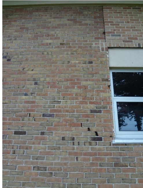
5. BROKEN + MISSING BRICK THROUGHOUT AREA OF FAÇADE - CLEAN & REPOINT MASONRY AS NEEDED. INSPECT ANNUALLY.
