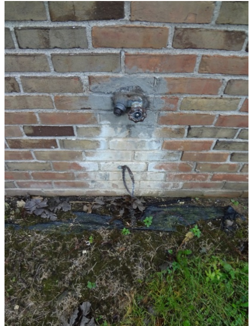
3. EXTERIOR WATER BIB, RESIDUE ON FACE OF BRICK INDICATES LEAKING WATER - CLEAN ORGANIC MATTER FROM BRICK, INSPECT WATER BIB AND REPAIR AS REQUIRED
