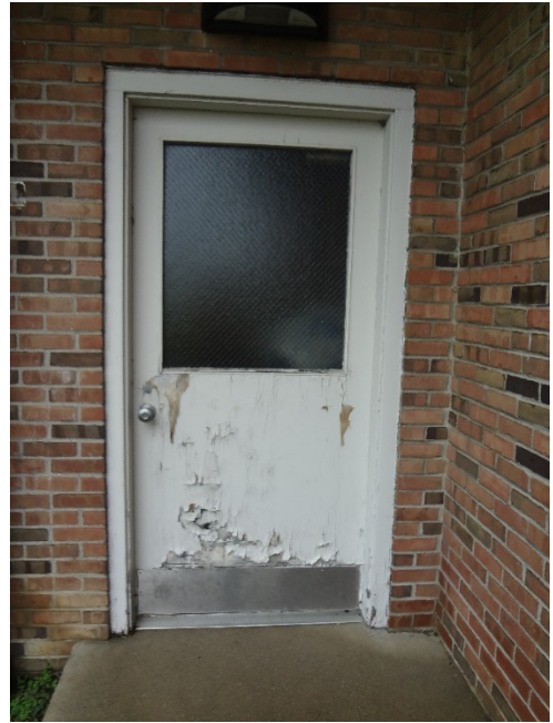
13. PEELING PAINT + DAMAGED WOOD SERVICE DOOR - REPLACE EXISTING WOOD SERVICE DOOR WITH NEW STEEL DOOR AND FRAME
